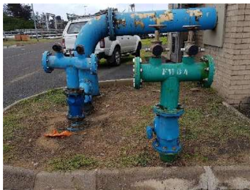
Figure 3-5: Pipe manifolds located outside of the foam pump station
