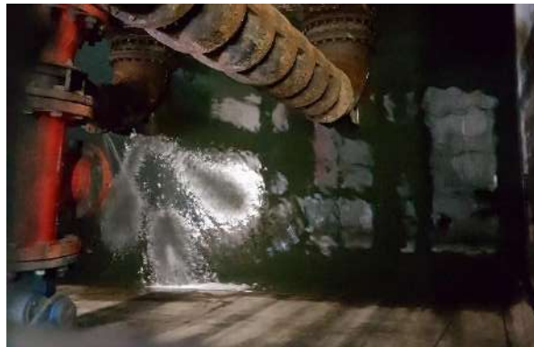
Figure 3-4: Intake sump showing multistage pump
