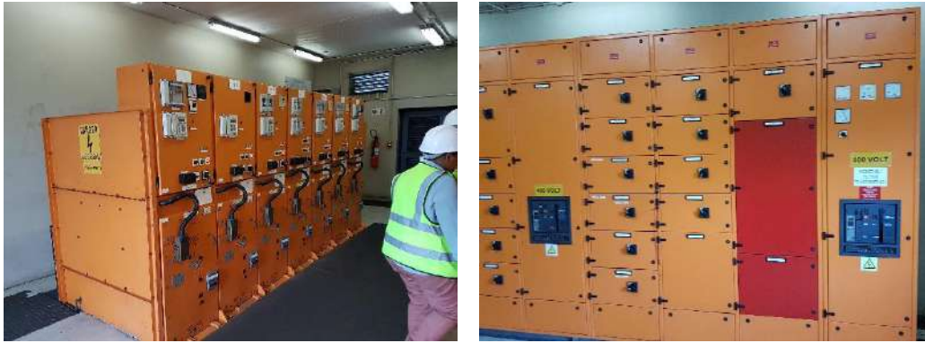
Figure 3-1: MCC & electrical panels in berth sub-station
