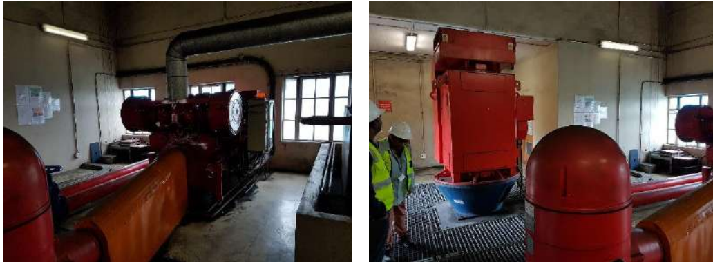
Figure 3-3: Seawater pump station
