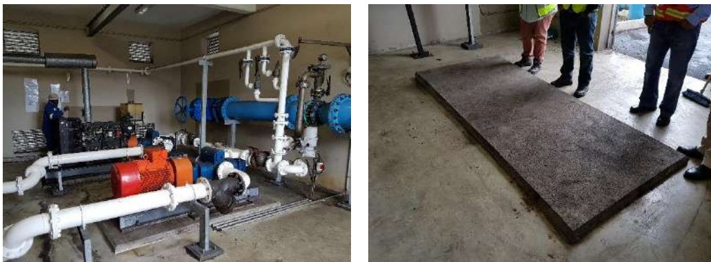
Figure 3-2: Foam pump station and spare base
