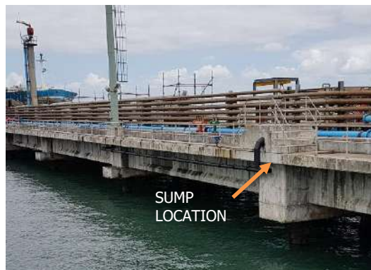
Figure 3-11: Stormwater Pump Sump
